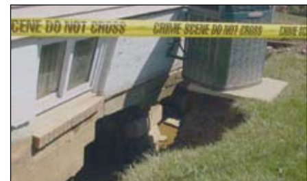
6. HYDROSTATIC PRESSURE COLLAPSES FOUNDATION WALL
