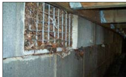
5. TYPICAL AIR VENTS CLOG WITH DEBRIS
